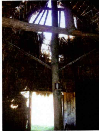
The damaged "ruka".
