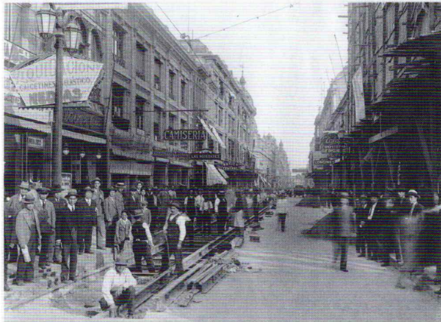
Calle Ahumada. Santiago entered the new century with electric trams. This photograph shows the installation of the tram rails.
